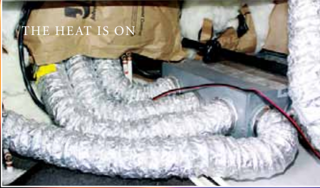
Inspect the flexible ducting for cracks or tears; use aluminum tape for any repairs. Also inspect any areas where the ducting may have become crushed or broken loose from the collars.
