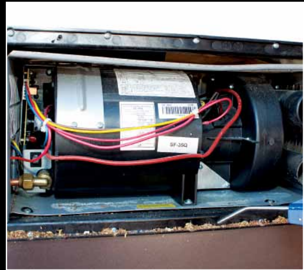
With the access door removed, inspection of all components can be quickly visualized. Clean out any excess dust, lint or, in this case, sawdust at the base of the door frame.
