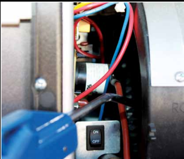
Accessing the Suburban furnace's blower wheel can be a challenge. However, it is important that area be cleaned on an annual basis using compressed air.
