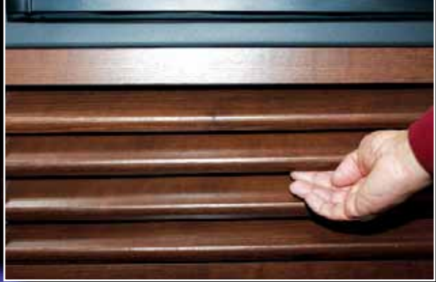
The interior return air vent must be clear of any debris for proper furnace function.
