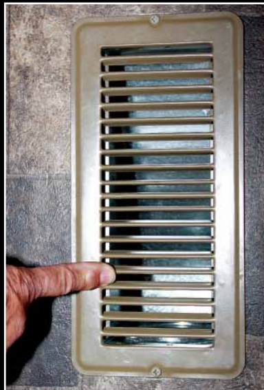
Remove the floor registers and vacuum out any lint, dust or debris to prevent buildup in the ducting system.
