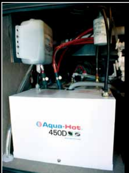
Be sure this compartment area is not used for storage as to protect the many hoses and wiring.
