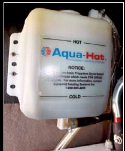
The antifreeze tank is mounted in a convenient location. Inspect the fluid level before every outing. If the fluid level is too low, it may indicate a leak in the system. Add fluid and check for leaks.
