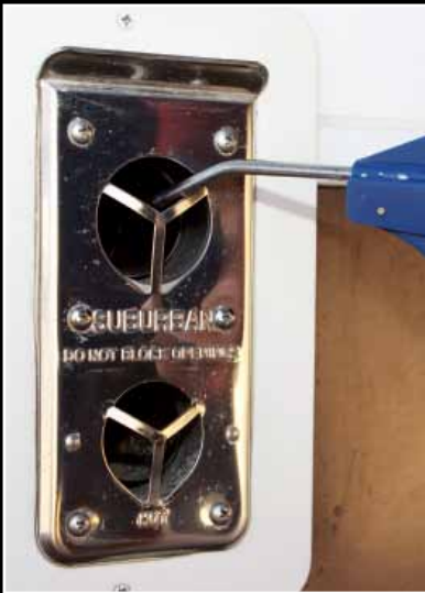
Using an air nozzle, blow air pressure through the intake and exhaust vents from the outside of the coach as part of the annual cleaning.
