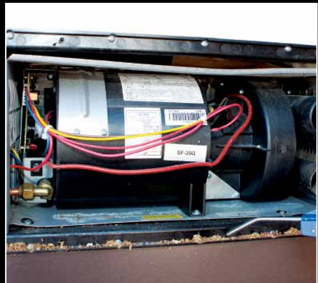
With the access door removed, inspection of all components can be quickly visualized. Clean out any excess dust, lint or, in this case, sawdust at the base of the door frame.
