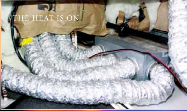
Inspect the flexible ducting for cracks or tears; use aluminum tape for any repairs. Also inspect any areas where the ducting may have become crushed or broken loose from the collars.
