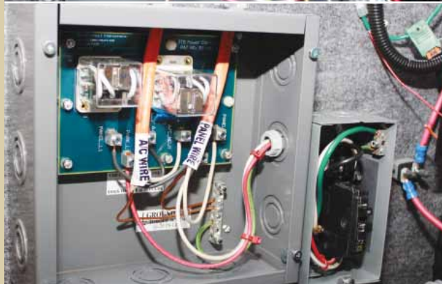
The JTB is mounted to a solid, vertical surface in a location close to the cable hatch exit for the JTB power cord. This gives the maximum amount of footage between the coach and campground power.
